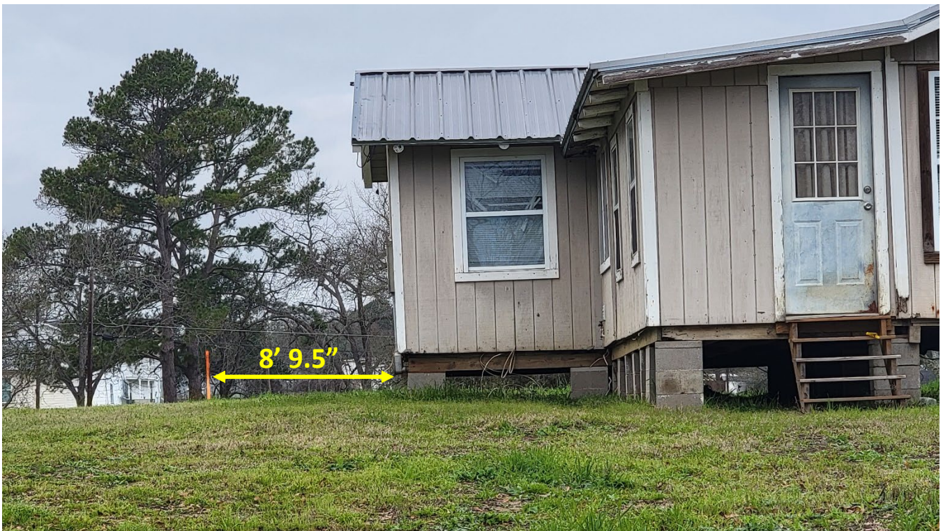
Encroaching south side – Survey stake shows the lot line.
